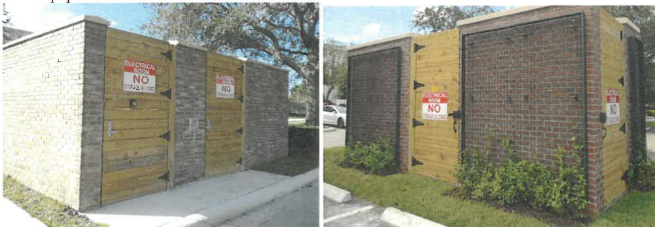
Tesla equipment enclosures at The Fountains
