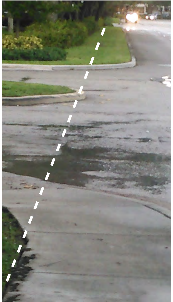
Exhibit 18. Missing Sidewalk Connection
