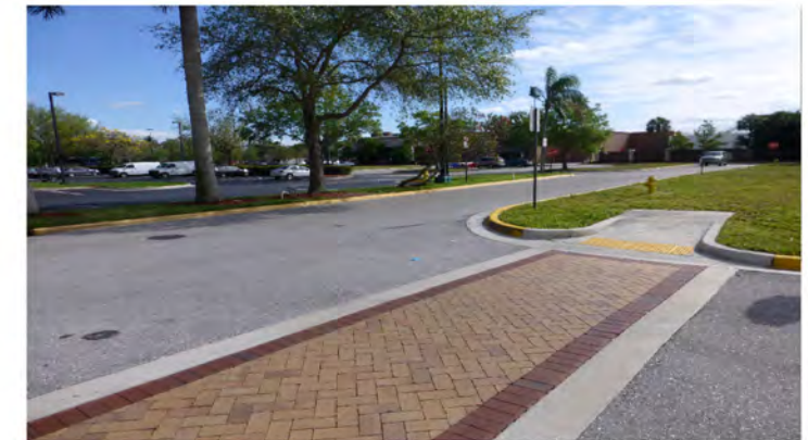
D) Sidewalks abruptly end, due to abutting private property
