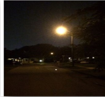
Existing HPS Street Light Fixture
